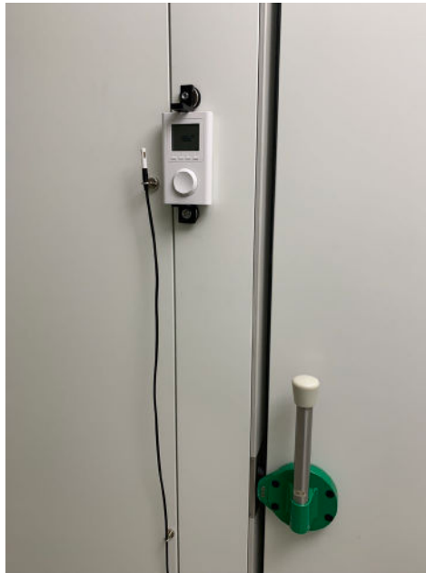
Figure 9: Room thermostat next to the door, including a reference measurement point
