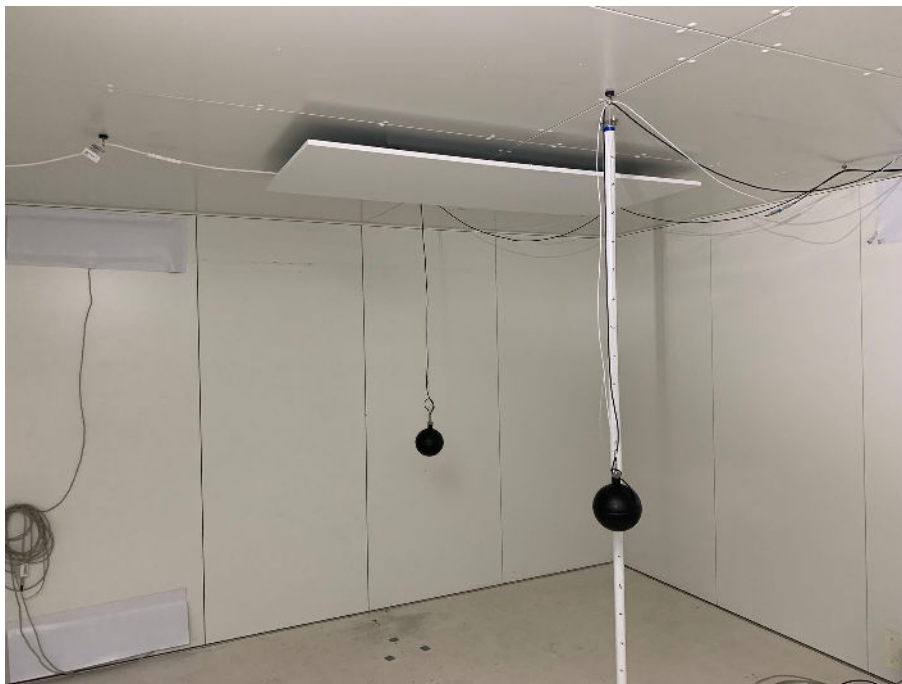
Figure 6: Infrared heating system mounted on the ceiling – near position
