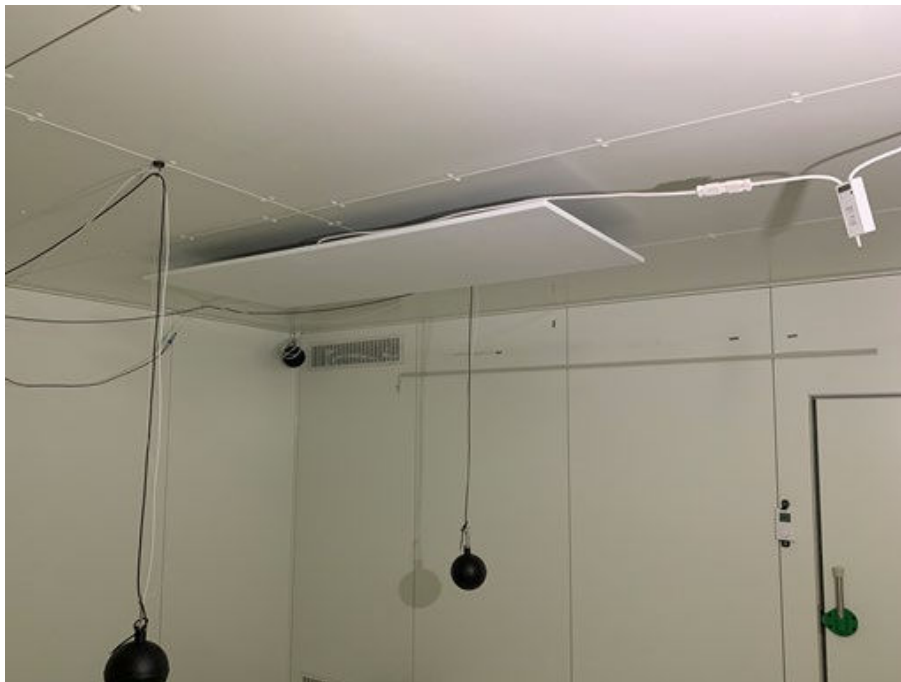
Figure 8: Infrared heating system mounted on the ceiling – far position
