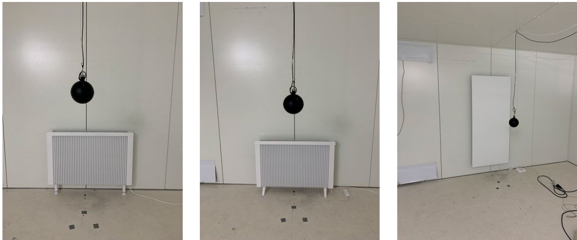
Figure 4: Heating units installed in the indoor climate room – Left: Dynamo heating system; Center: Partial storage heating system; Right: Wall-mounted infrared heating system
